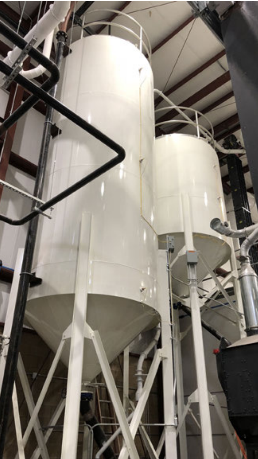
Bulk aggregate storage system
